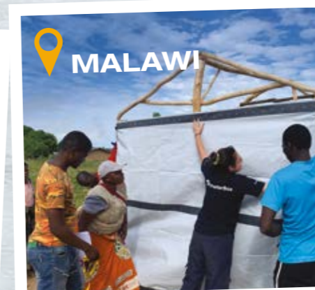
MALAWI After the flooding in the Nkhotakota district of Malawi, the team held an artisan training and demonstration session. Tarpaulins were used for the walls and roofing of the local wooden framed structures.
