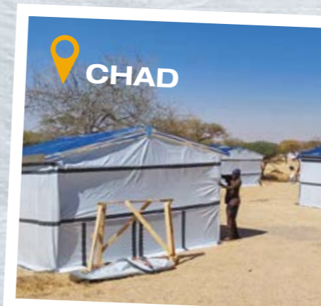
CHAD We provided tarpaulins and fixings for the construction of transitional shelters for refugees in Chad. In a joint project with UNHCR, these shelters used tarpaulins as the exterior material across a timber frame with a corrugated iron roof.
