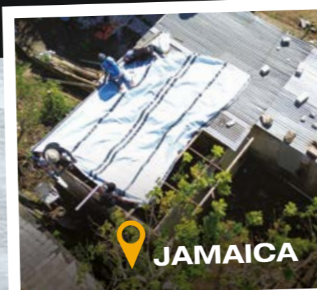
JAMAICA Islanders on Jamaica needed to quickly seal their roofs after they were destroyed by Hurricane Melissa. Tarpaulins were used in a number of ways, sometimes to simply provide a waterproof barrier to further rainfall.
